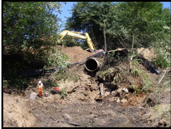
FIGURE 1. Estero road culvert at Point Reyes National Seashore. Though partially obscured by shadows, an eroded, drippy, wet cavern is visible on the underside of the culvert. The cavern appeared to be ideal salamander habitat. When the culvert was lifted, 27 Dicamptodon ensatus were exposed, along with other amphibians and reptiles (Table 1).
